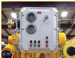
NEMA 7/9 CONTROL PANEL
